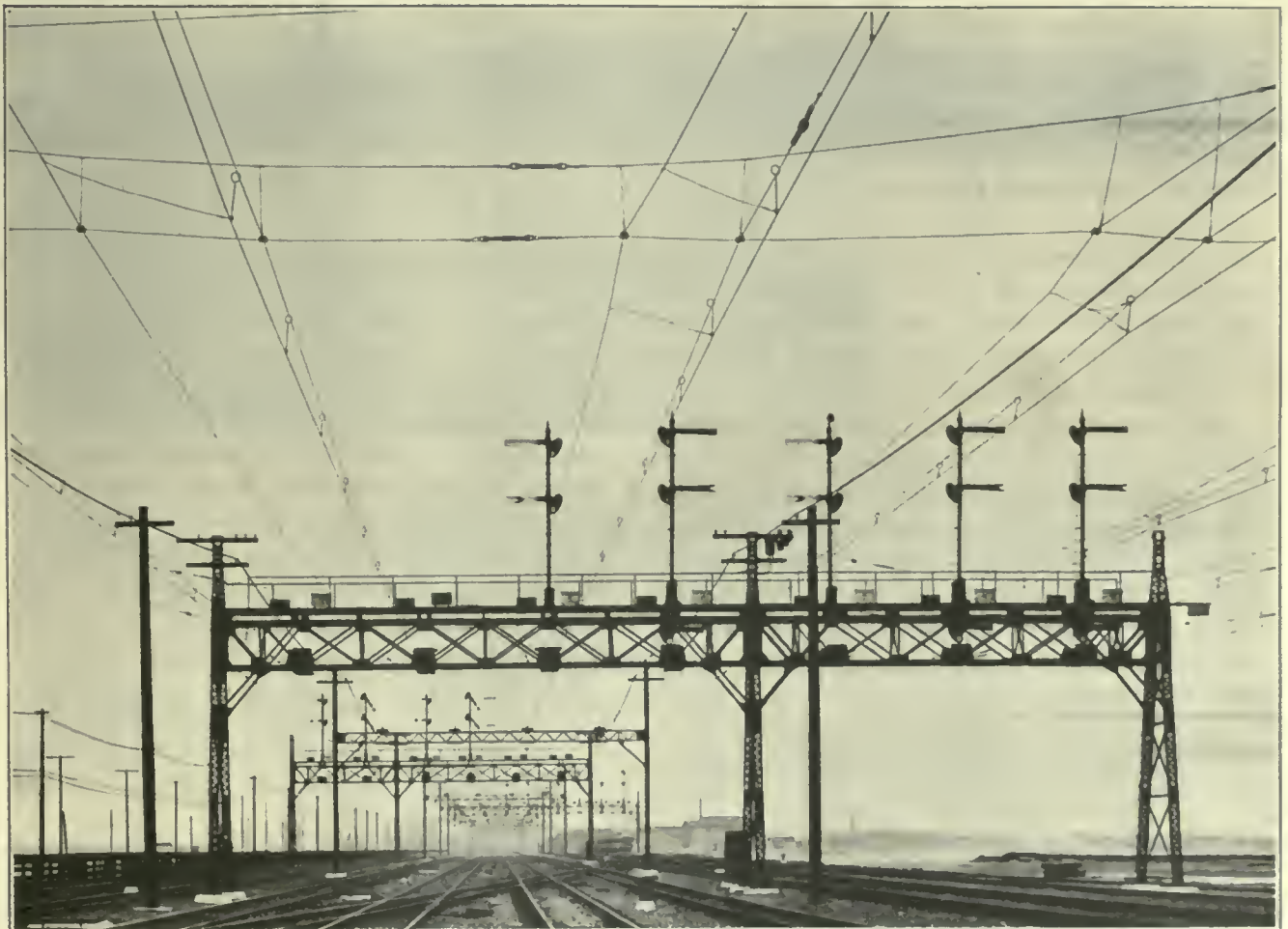
FIG. 526. OVERHEAD CONTACT SYSTEMS. Catenary Construction, 1,200-Volt Direct Current Main Line, Southern Pacific Railroad, near Oakland, Cal.
